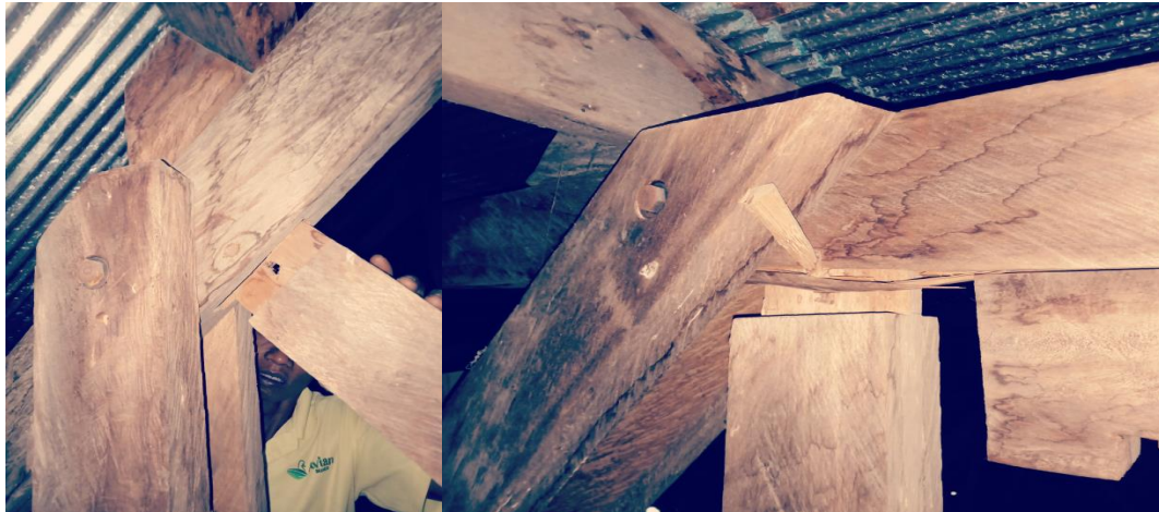
Fig. 2. Damages of Timber Joints of Timber Truss of Sigi Regency
