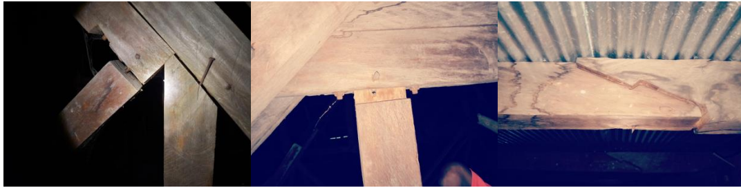
Fig. 1. Damages of Timber Joints of Timber Truss of Sigi Regency
