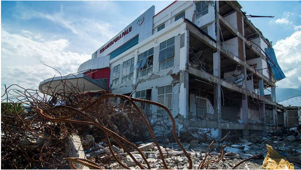
Figure 1. Structural failure and foundation settlement of RSU Anutapura induced by post-liquefaction effects following the 2018 Palu Earthquake
